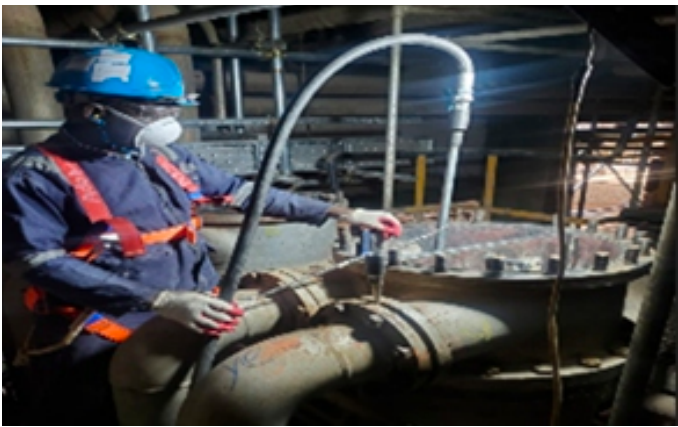
Air Blowing for Heat Exchanger
