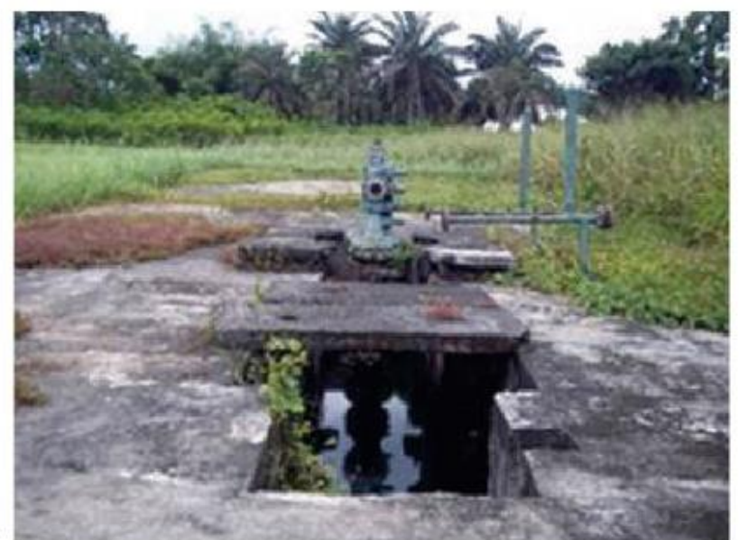
Fig 2: ASSA oil wellhead (dual string)
